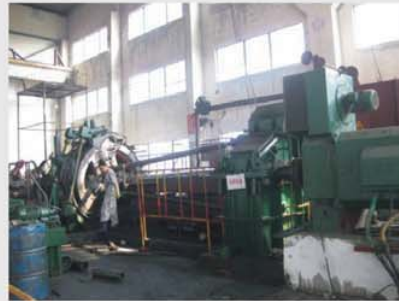
无缝管材轧制设备 Rolling equipments for seamless pipe materials
